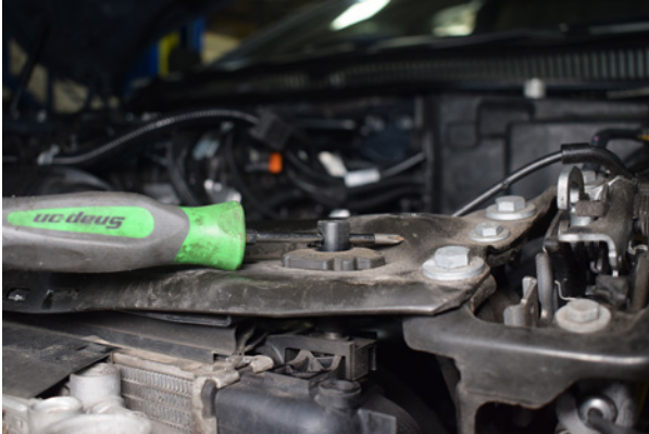
43. Before going any further, place a screwdriver/or similar into the radiator mounting point to stop everything falling.
