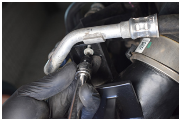
59. With the boost hoses connected relocate the mounting screws to secure the intercooler to the car. Repeat on both sides.
